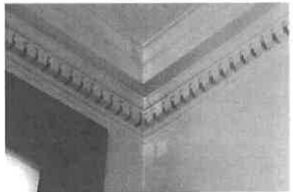
Lewes resident Shawn Swider picks up mail from his vintage post office box. Dentil molding along the lobby ceiling is a testament to the grandeur of civic architecture. Postal workers Joe Panzer and Donna Atsidis, on facing page, offer customers friendly, efficient counter service.
